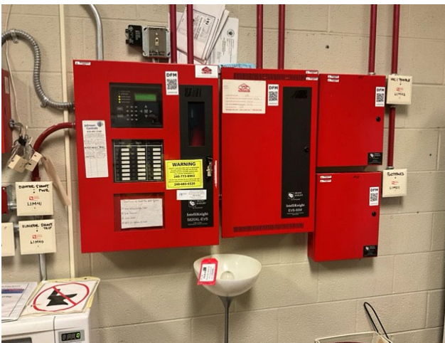
23 - FIRE ALARM PANEL
